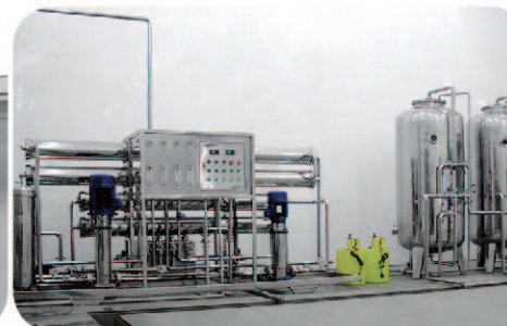
湖北黄石欧郎药业(5m 3 /h 二级反渗透纯化水设备) Hubei Huangshi Langou Pharmaceutical Co.,Ltd (Capacity 5m 3 /h two stage Reverse Osmosis equipment)
